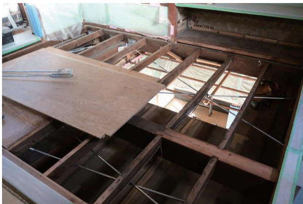
Installation of horizontal under-floor braces on the second floor (House of Koide)
