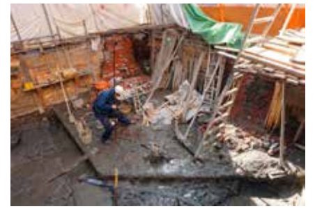
Pl. 2 Original tiles and octagonal foundation that emerged during a house construction project in February 2018 (Photo by the author)
